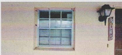
Unprotected glazed opening
