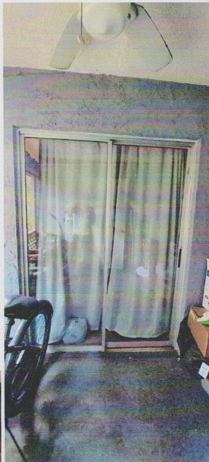
Unprotected glazed entry door
