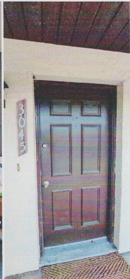
Unprotected non-glazed entry door
